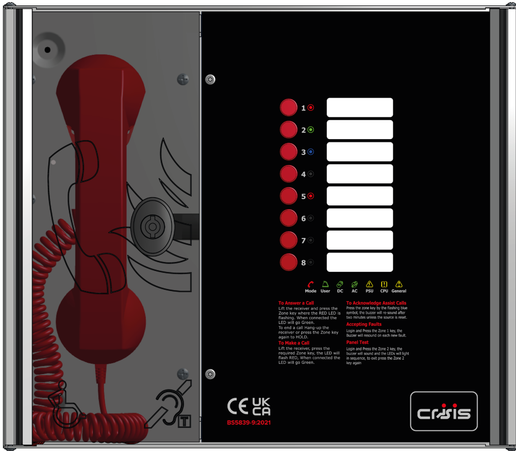
Figure 1: Crisis EVC Standalone Master Station Indication and Control
